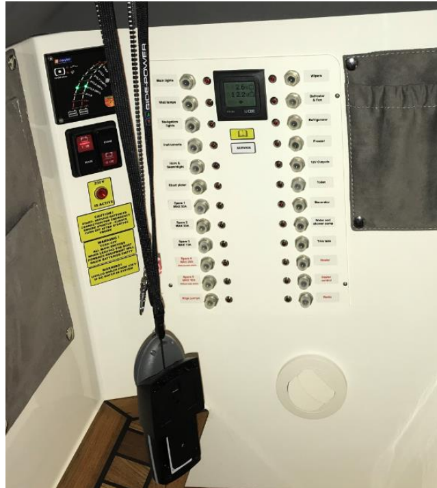
Picture 39: The fuse panel
