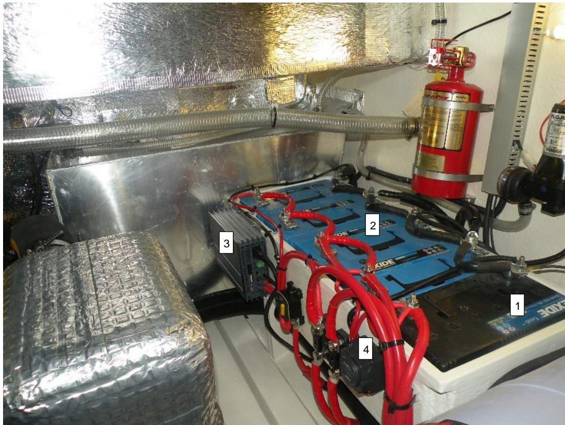
Picture 30: Starter battery (1) Service batteries (2) – Optional 4 items (Standard: 1 starter and 3 service sulphuric acid batteries) Battery charger (3) Dual sense charging relay (4)
