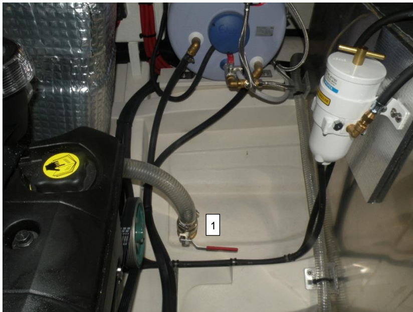
Picture 14: Location of seawater inlet for engine cooling and valve (1)
