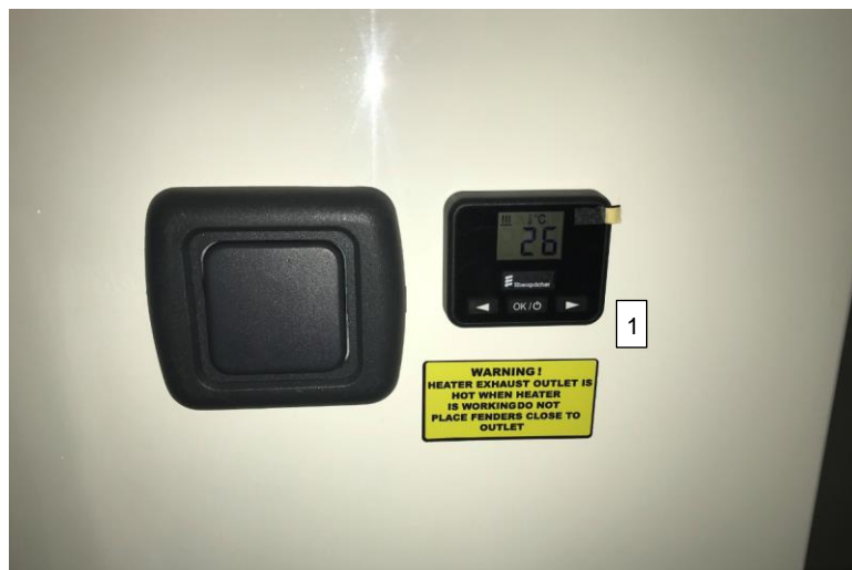
Picture 54: The heater switch (1)
