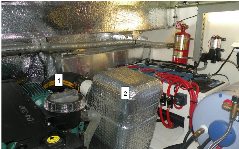
Picture 32: The exhaust hose (1), water lock muffler (2)
