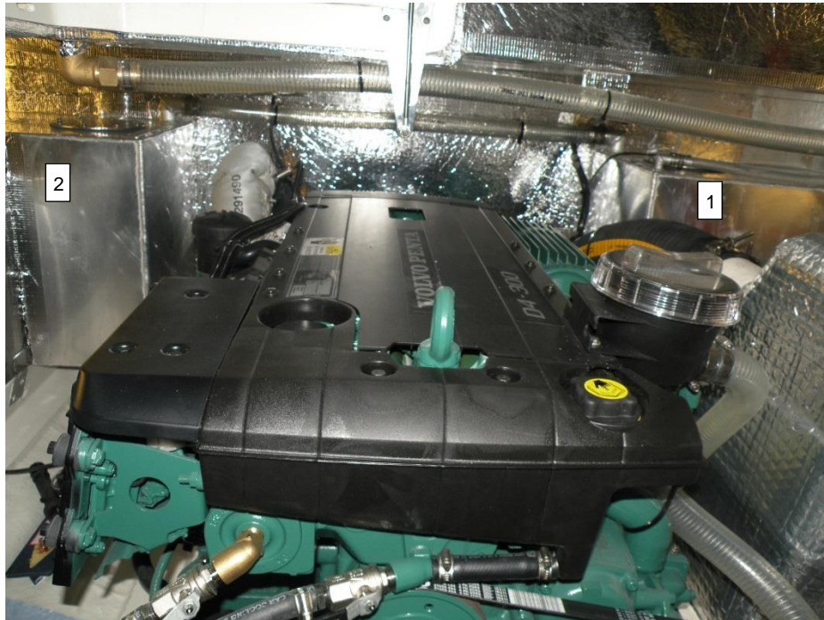
Picture 25: Fresh water tank in the engine room – port side (1), fresh water tank – starboard side (2)
