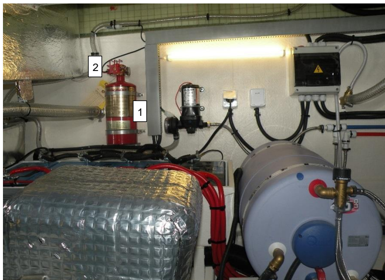
Picture 35: Automatic fire extinguisher in the engine room – 2.5 kg capacity (1), fire extinguisher volume level (2)
