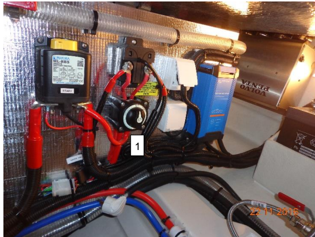
Picture 38: Batteries crossover switch (1).
