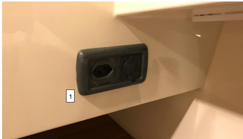
Picture 45: 230 V socket in the front cabin near the main closet (1)
