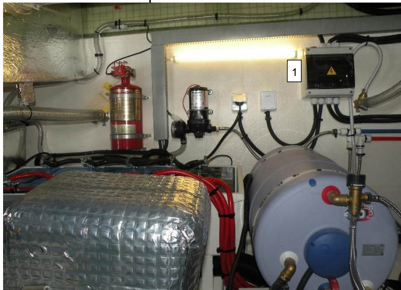
Picture 31: 230 V Main fuse 20A and grounding relay (1) (Lamp indicates when 230 V is active.)
