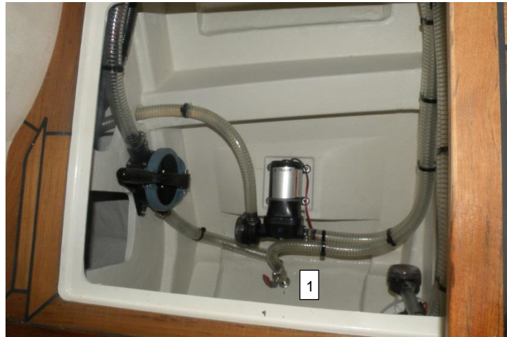
Picture 11: Location of the seawater inlet for the toilet flush (1)
