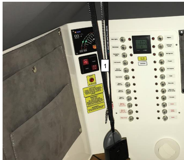
Picture 40: Main switches (1)
