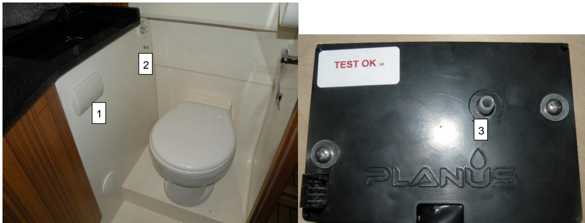
Picture 27: Toilet controls (1), ventilation (2), water level trimmer shaft
