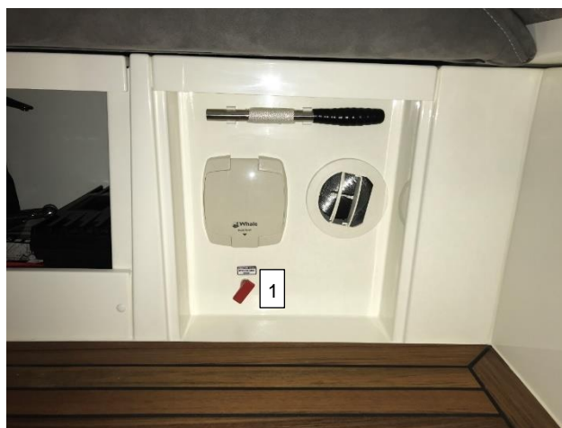
Picture 9: Emergency engine fuel closing valve and extinguisher with engine stop – sitting group (1)
