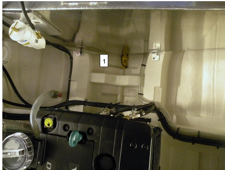
Picture 59: Pump inlet in the engine room (1)
