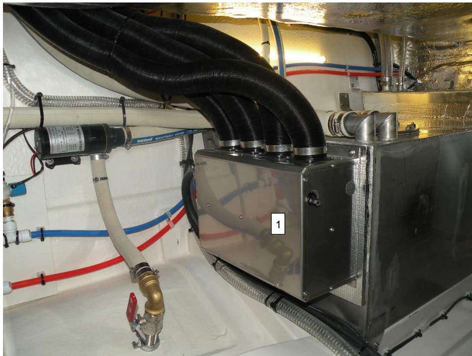
Picture 52: Defroster location in the engine room (1)
